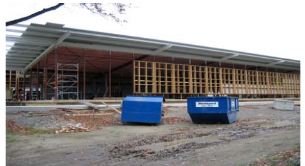
Using 2 skips to sort recycling and landfill waste at South City Library, Christchurch (Mainzeal)
